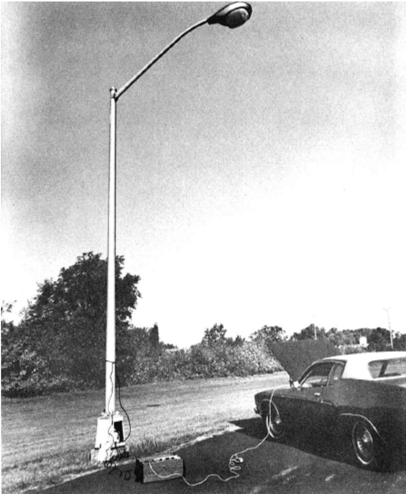
Figure 5: Testing Parking Lot Lighting; the Test Set Shown is Operating from an Inverter.
